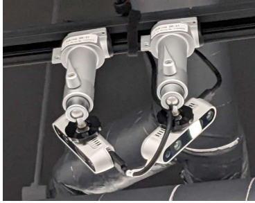
図 3: Ceiling mounted Intel RealSense Cameras
